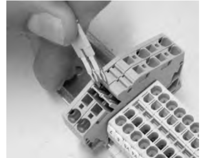
Remove shunt to deactivate a heater (reduction of 300 W)
